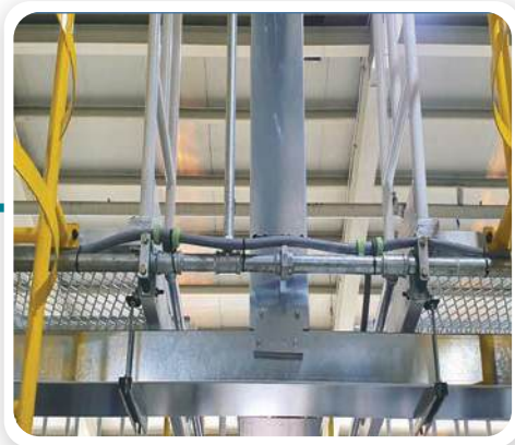
03 Image connecting the PB piping
