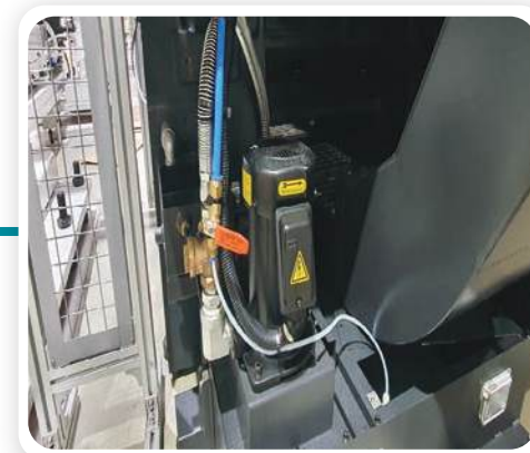
05 Image of connecting ball valve to urethane hose (12A) and connecting ball top to processing equipment
